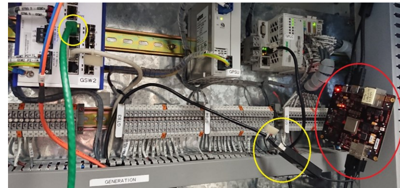
BITW device integrated into EPIC Testbed
